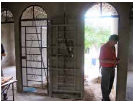
Peter Yau examines construction at the National Presbyterian Center near Santa Clara.
